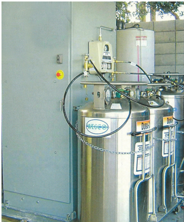
Mobile ozone/peroxide pilot treatment system.
